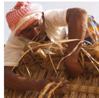
Date palm leaf house with external palm panels, using rope made of palm hair from the top of the palm's trunk
