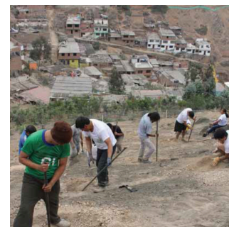
The plantation efforts also secure the safety of the residents at the hillside.
